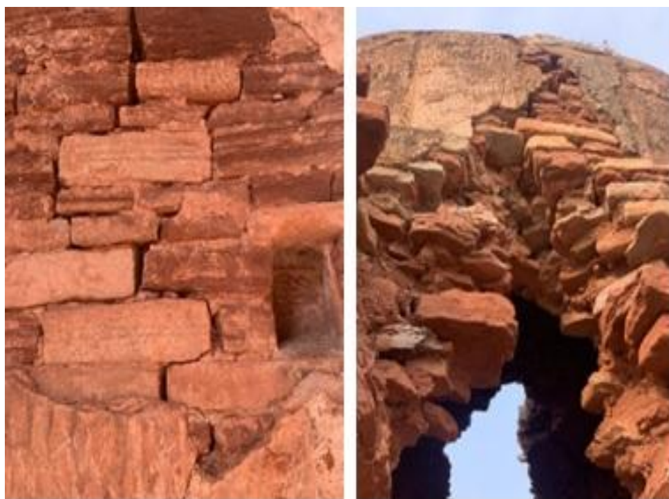
Figure 7 Damage to the structure
