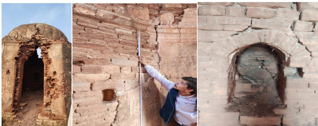
Figure 2 Structural Deterioration and Material Loss
